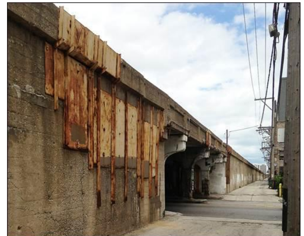
(Above right) Crumbling viaduct at Hollywood Ave. between Bryn Mawr and Thorndale Stations
