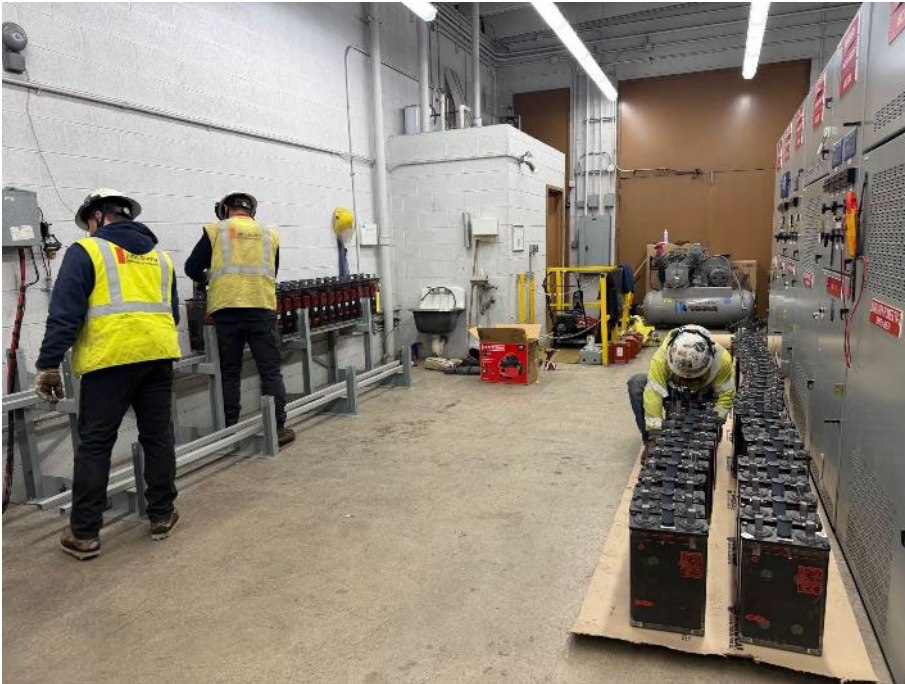
Backup Battery Installation at Damen
