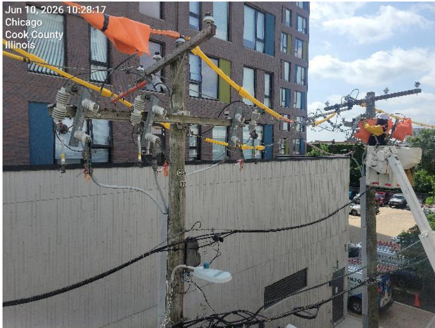
ComEd – Isolation of Station Power Transformer
