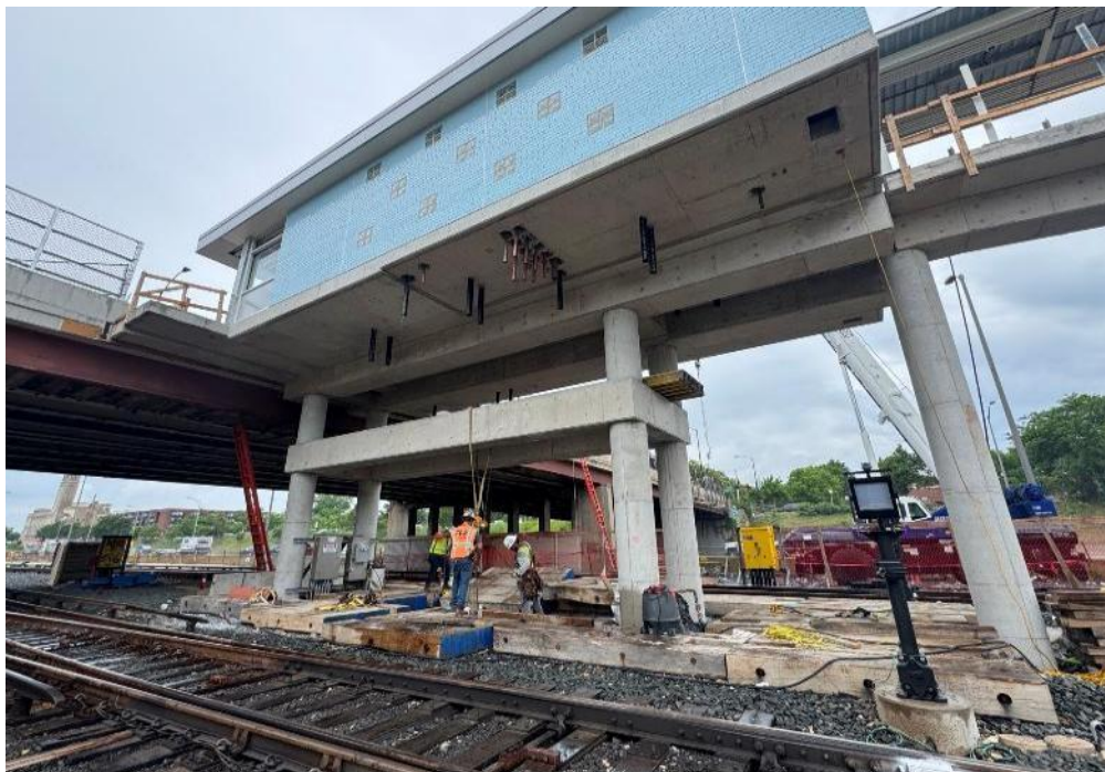
Loomis Stationhouse Exterior Plumbing
