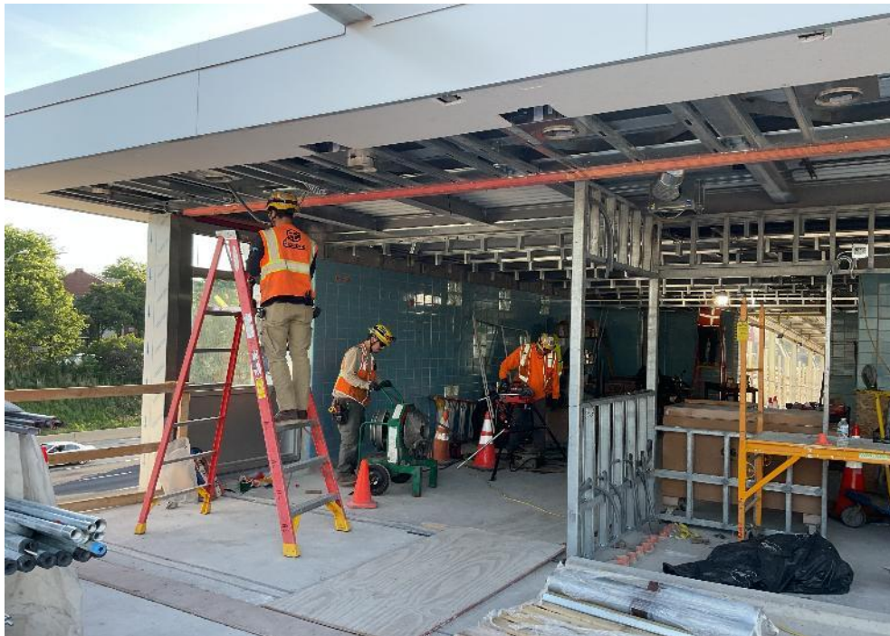
Loomis Stationhouse Ceiling Electricals
