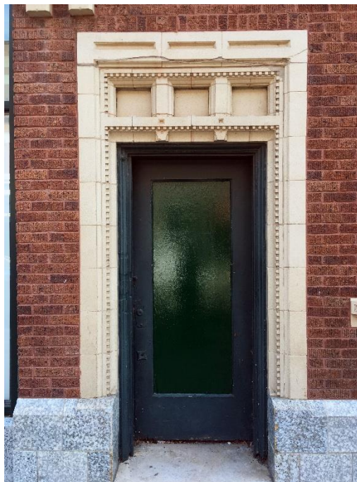
Example of a historic residential entry door in the district, with an intact, original opening.
