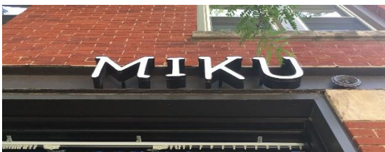
Example of inappropriate sign mounting, located outside of the district, as the sign is directly attached to the historic cast iron header.
