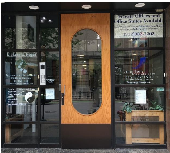
Example of an inappropriate contemporary replacement door and opening not in the district.
