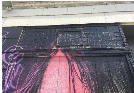
Example of historic prism glass storefront transom, evident under the paint, in the district. Prism glass was introduced in the 1890s as a popular and practical way of directing daylight into building interiors. The glass had ridges or other raised patterns on the inside surface that refracted sunlight toward the rear of the building.
