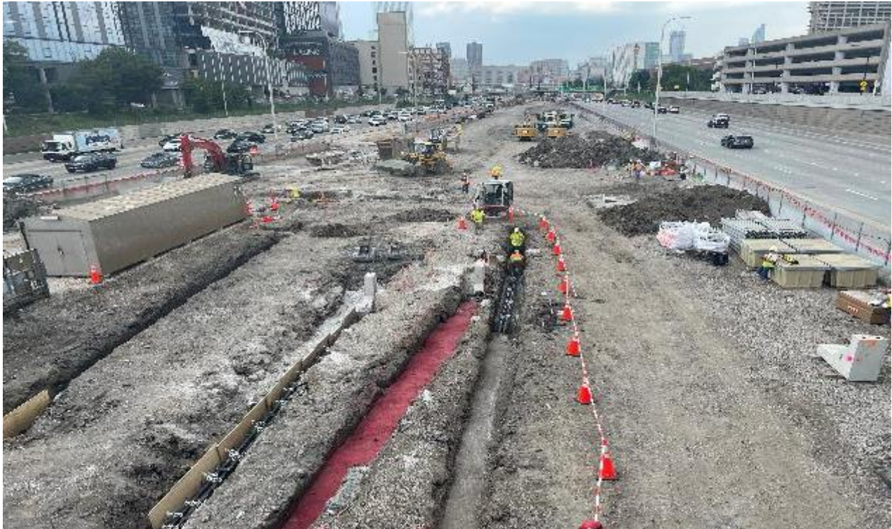
Duct Banks East of Racine
