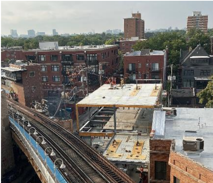
Birds Eye of Damen Substation
