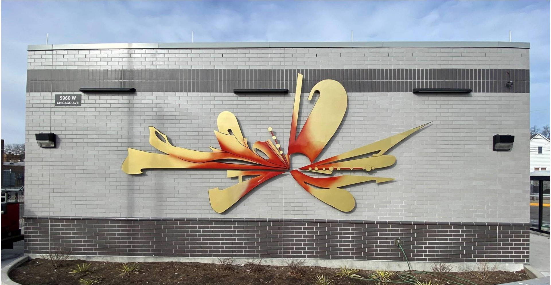
Electric Substation for Charging Pantograph and Artwork Chicago and Austin Bus Terminal
