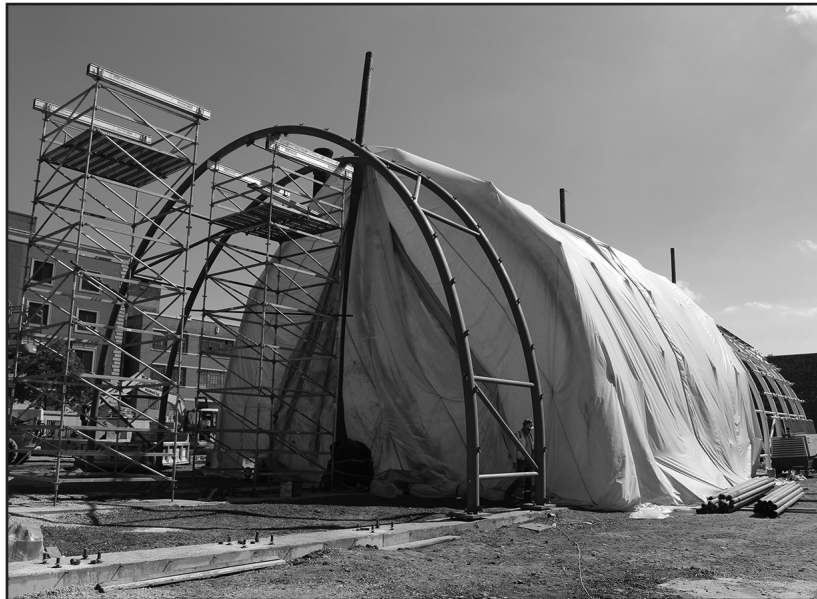
Crews pre-assemble steel tubing that will be lifted into place with cranes to create the tunnel covering the tracks and platform area of the new Cermak-McCormick Place Green Line station.
