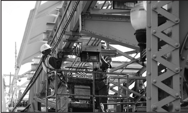
The CTA's historic project labor agreement promotes employment opportunities to disadvantaged workers on many projects, including Your New Blue renovation work at the California station.
