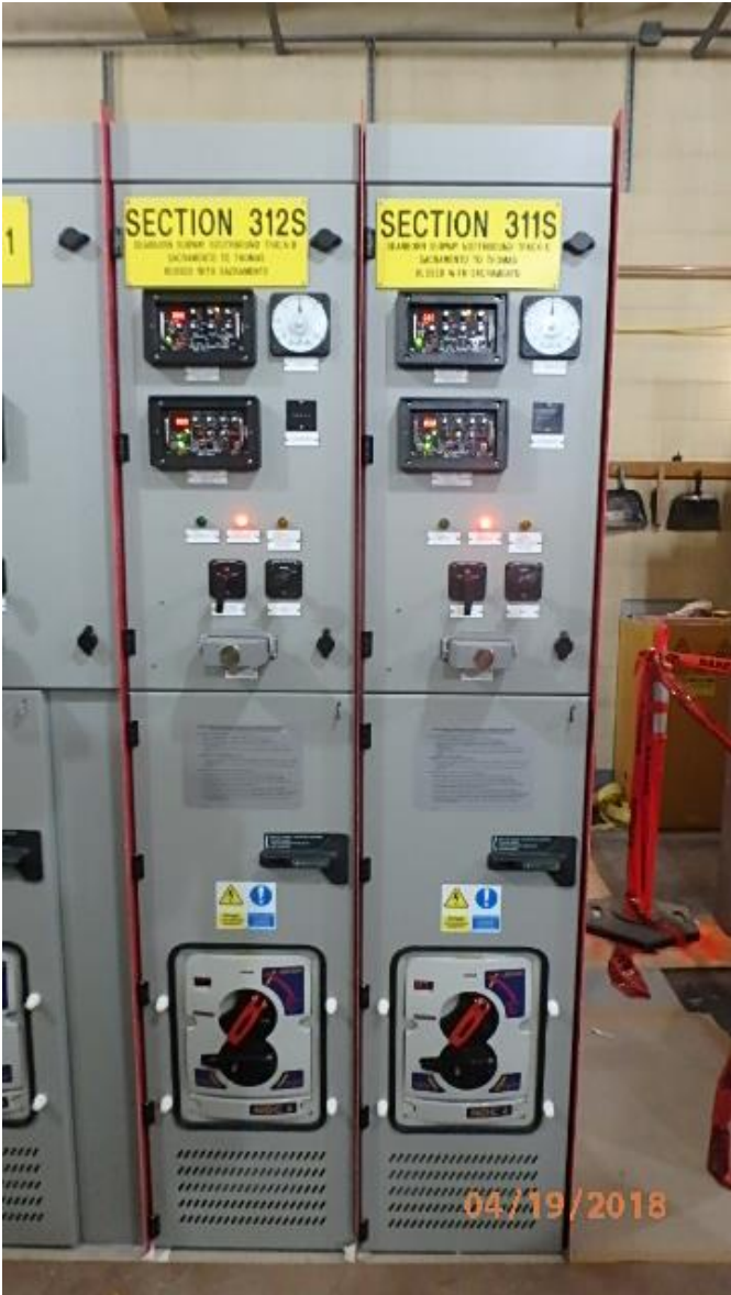
Milwaukee Substation - New DC Breakers
