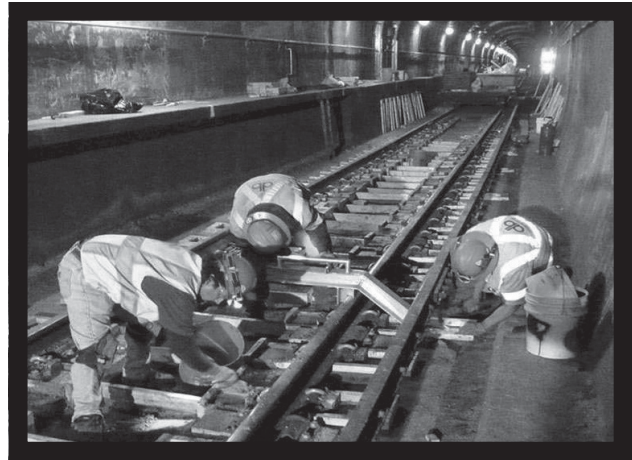
Crews work to replace rail ties, running rail and contact (third) rail to remove emerging slow zones and help prevent the creation of new slow zones in the Blue Line's Dearborn subway.
