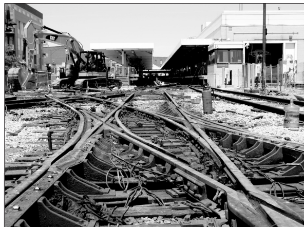
This summer, the Kimball Brown Line terminal was closed for nine days to replace track and rail system components that were 50 years old and beyond their useful life.
