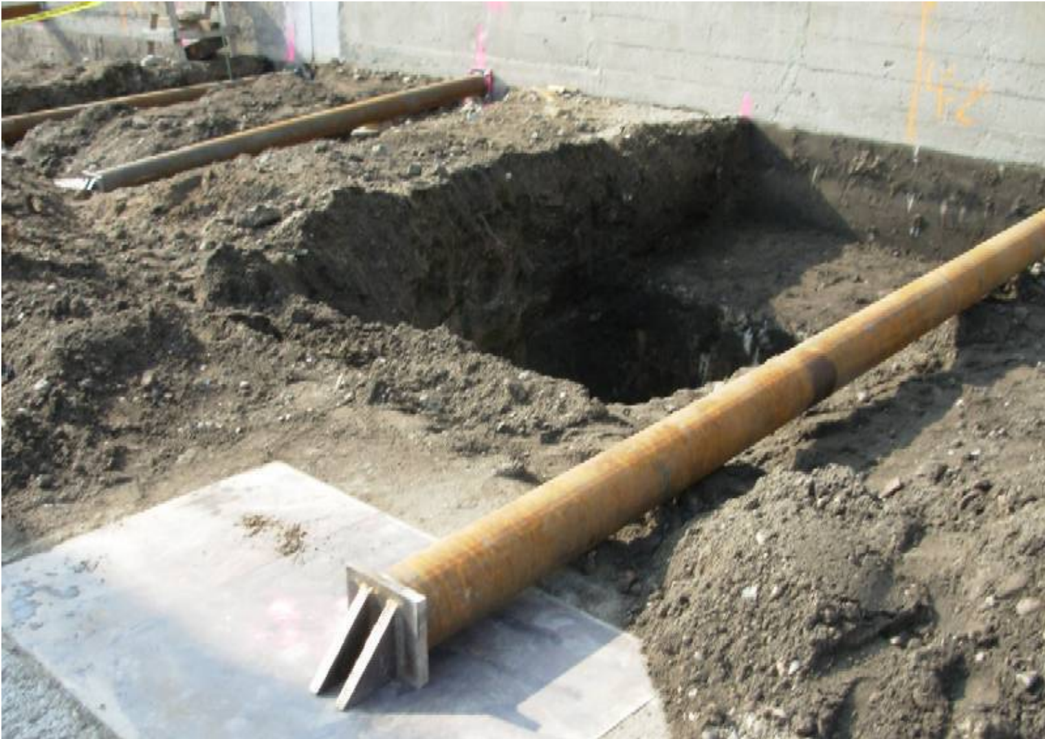
Lateral bracing system on east retaining wall
