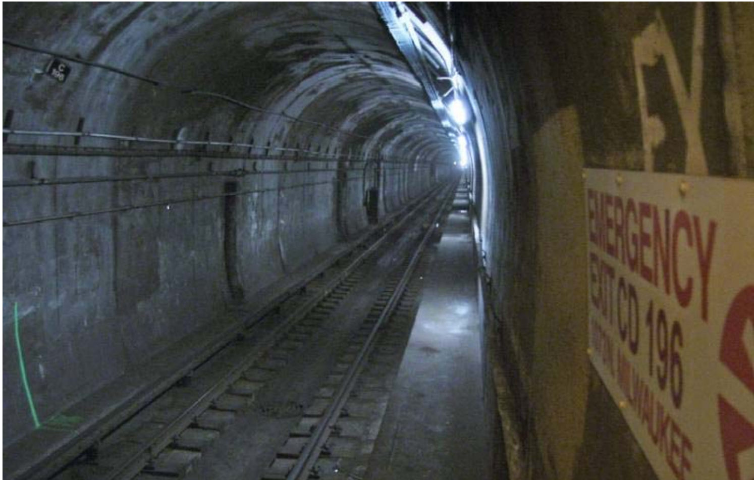
New lighting fixtures – Dearborn Subway
