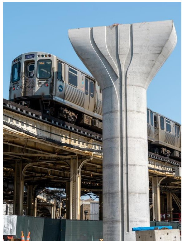
One of several new support columns erected next to the Purple Express Line tracks as part of RPM Phase One’s Belmont Bypass project.
