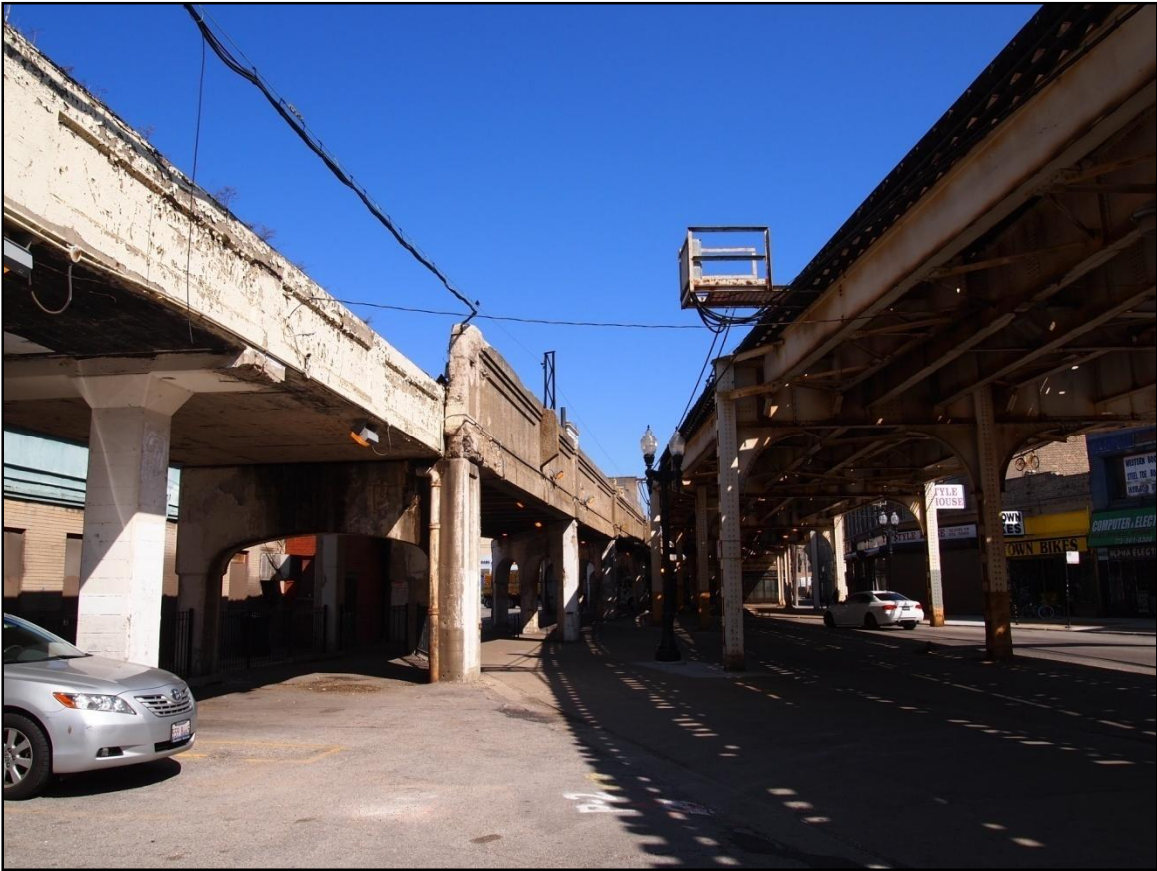
Plate 13. Convergence of concrete freight line and steel passenger line on the west side of N. Broadway Avenue and north of Wilson Station, view north.
