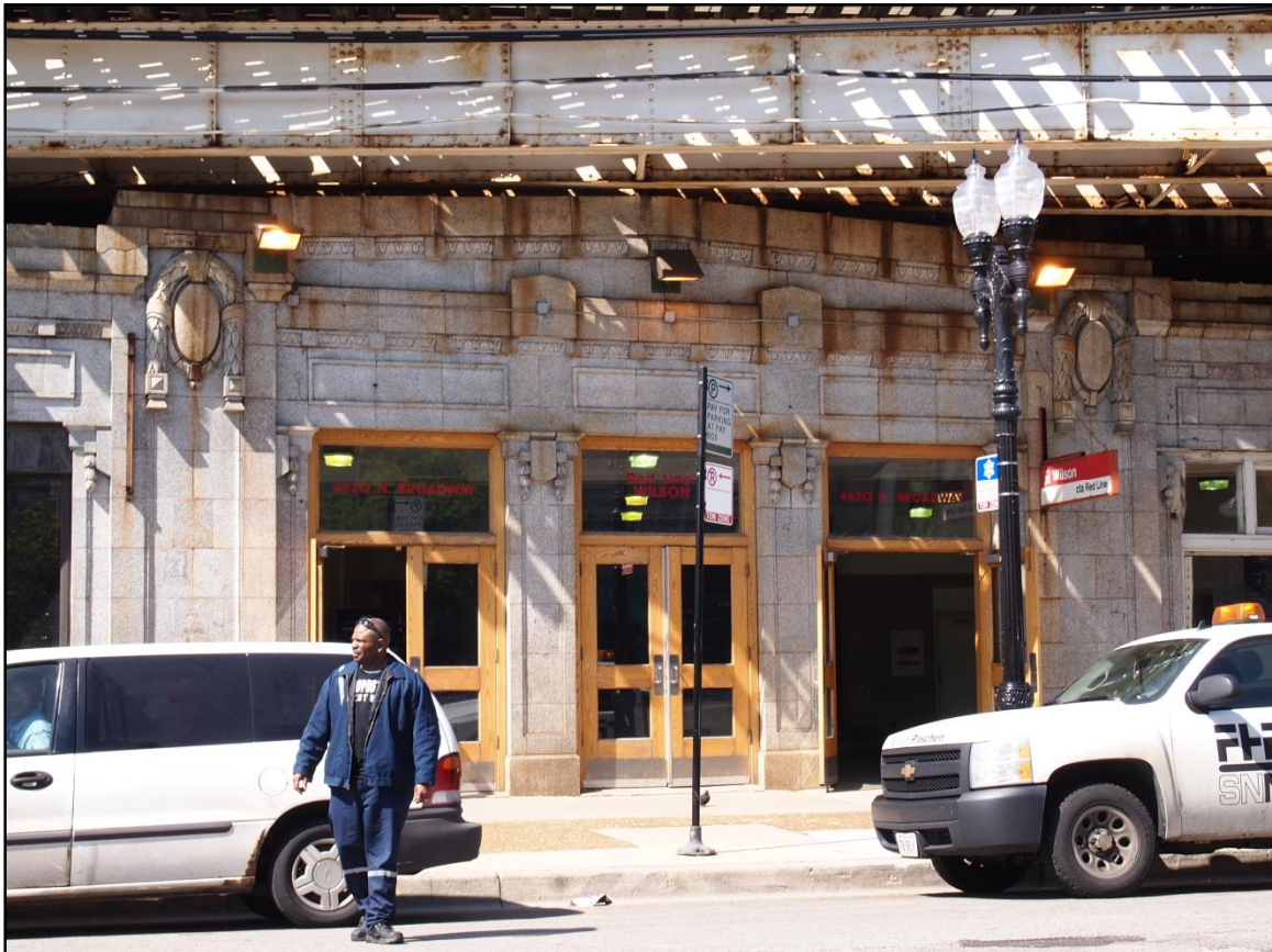
Plate 20. Main entrance of Wilson Station on east elevation (N. Broadway Avenue), view west.
